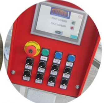
The Control Panel Kumanda Paneli
